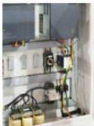
Electric appliance unit
